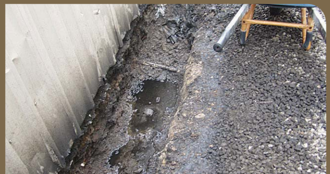
FIGURE 30: COMPLETELY NON-COMPLIANT WORKSITE, OILS, FUELS AND OTHER VEHICLE FLUIDS LEAKING INTO UNSEALED PIT
